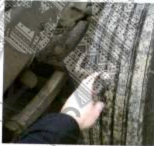
b. (1) Air line Obstructed
