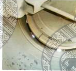
g. (1) Brake Drum Cracked
