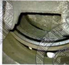
a. (5) (c) Contaminated Brake Lining
