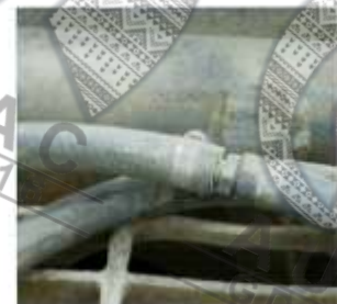
h. (4) Brake Hose Improperly Joined
