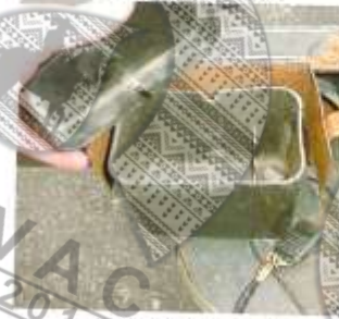
d. (1) Missing or Inoperable Breakaway Device
