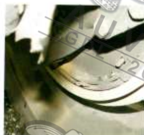
a. (5) (c) Brake Lining Void
