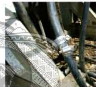
h. (4) Brake Hose Improperly Joined
